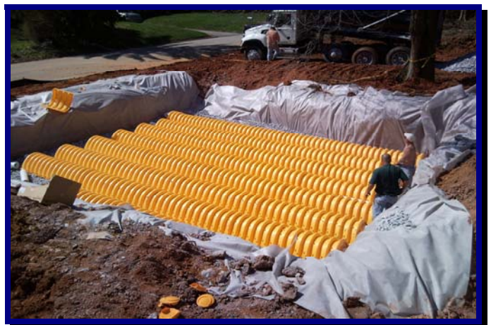
Subsurface infiltration system for stormwater management and groundwater recharge. System was tested and designed by Hagerty
