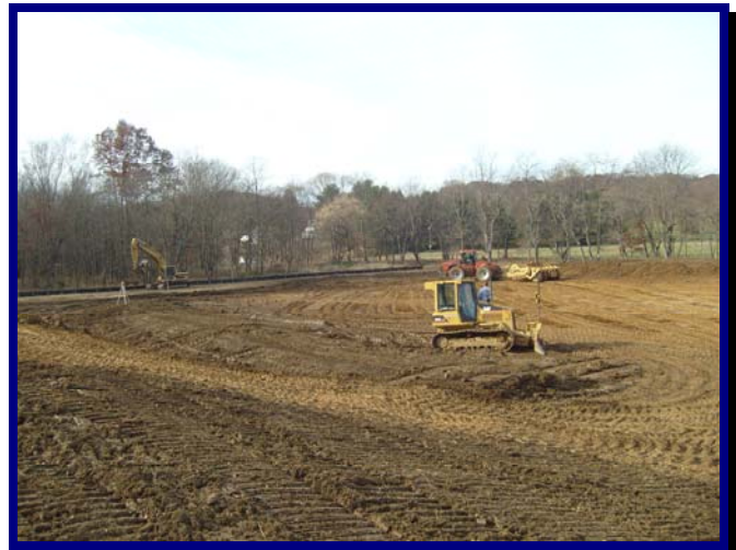
Five (5) acre waterfowl habitat pond being constructed in Northern Delaware. Hagerty provided design and construction oversight services for this project
