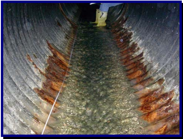
Inspection of a dam's primary outlet structure. Degradation of the CMP resulted in an emergency drawdown order from PADEP and the repair/reconstruction of the dam. Hagerty provided design and construction management services for this project
