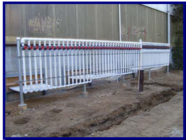
Air sparge/soil vapor extraction (AS/SVE) system manifold installed to address chlorinated solvents in soil and groundwater
