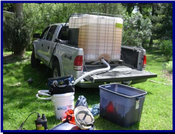
Subsurface injection of microorganisms and nutrients to enhance biodegradation of a fuel oil release below an occupied structure
