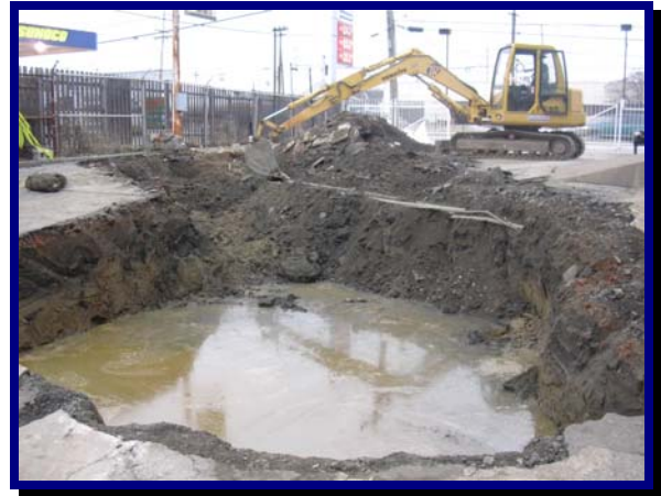
Petroleum-impacted soil excavation resulting from a leaking underground storage tank
