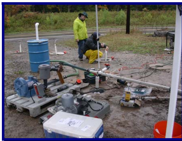
Pilot test of an air sparge / soil vapor extraction remediation system at a UST release site
