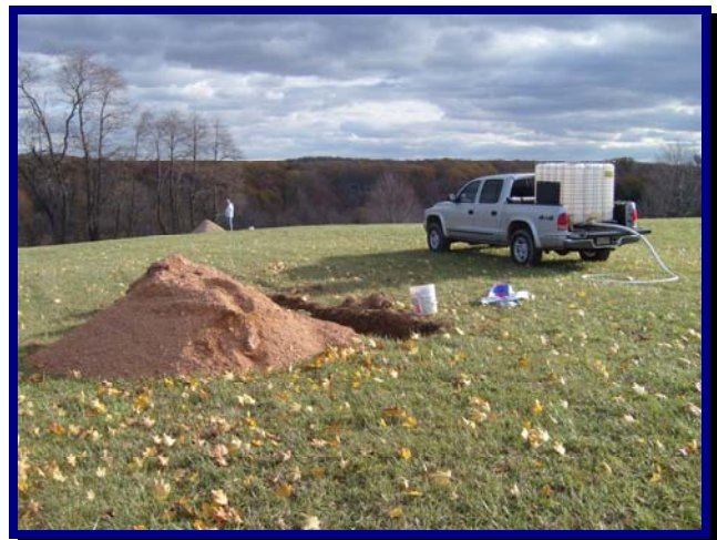
Hagerty provides stormwater management testing and design services, such as stormwater infiltration testing (shown above), in support of a Low Impact Development (LID) process. Subsequent services include subsurface infiltration BMP design
