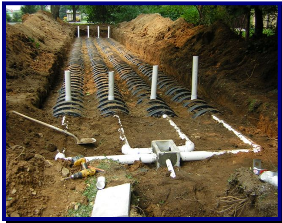
On-Lot sewage treatment system using leaching chambers
