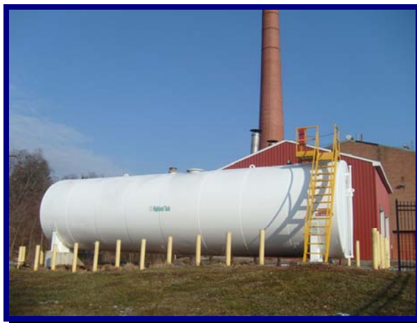
40,000 gallon dual-containment AST at facility requiring an SPCC Plan
